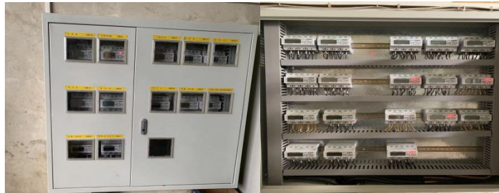
Electricity meters installed for each process in Kyowa-GSK
